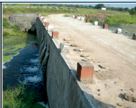
Plate 5. Spill over flow during tube well recharging
