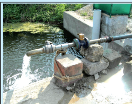
Plate 3. Submersible Pumping system with flow control valve and water meter arrangement
