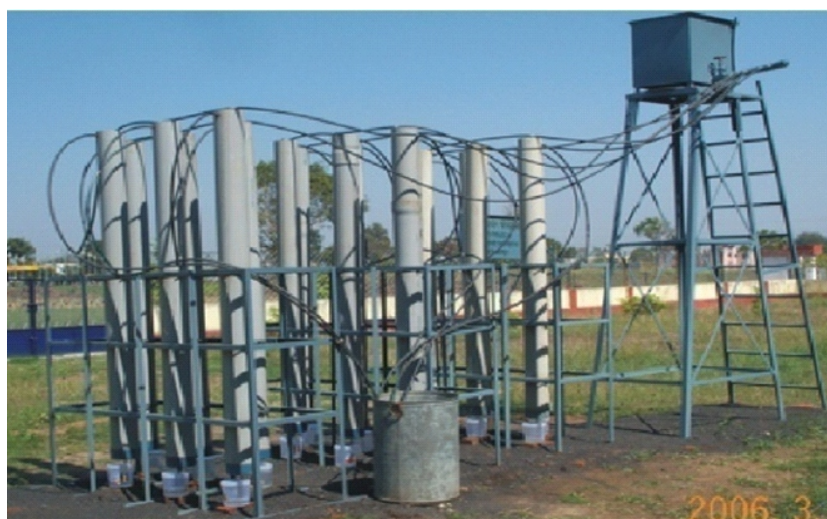
View of soil aquifer treatment plant
