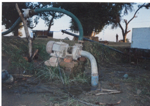
Loose foundation of the pump at farmers field
