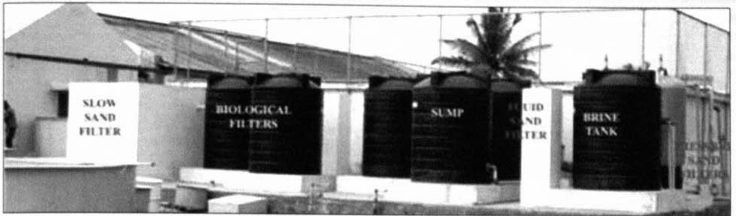
Seawater recirculation system
