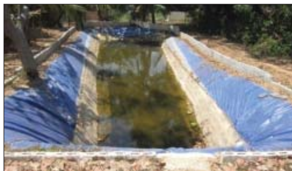
FLD on Lined tank
