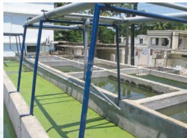
Effluent treatment plant
