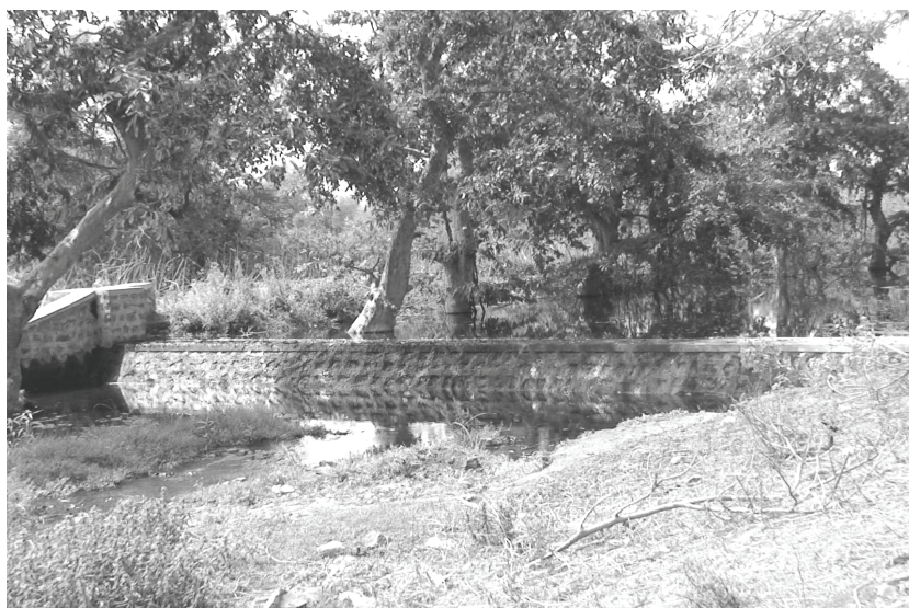
Photo 4 Concrete checkdam constructed and maintained with labour and money contribution of beneficiary farmers for soil and water conservation in Dahegaon watershed cluster of Vidarbha region of Maharashtra, India
