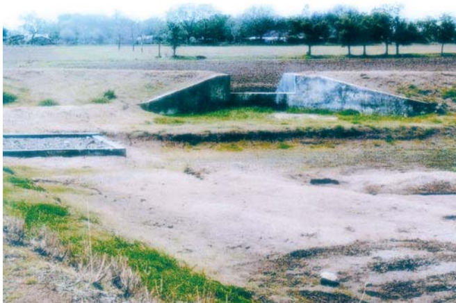
Recharge filter – A cost-effective technology for augmenting groundwater in arable and non-arable lands in the arid and semi-arid regions of Gujarat and Rajasthan
