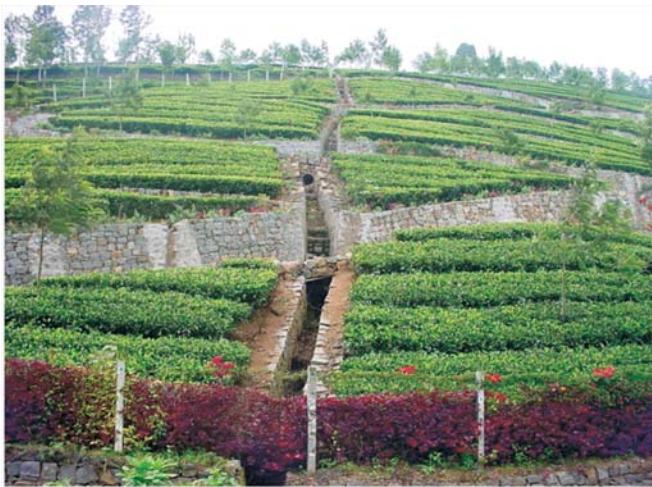
Vertical drain in tea plantation for safe disposal of runoff in the Nilgiri hills
