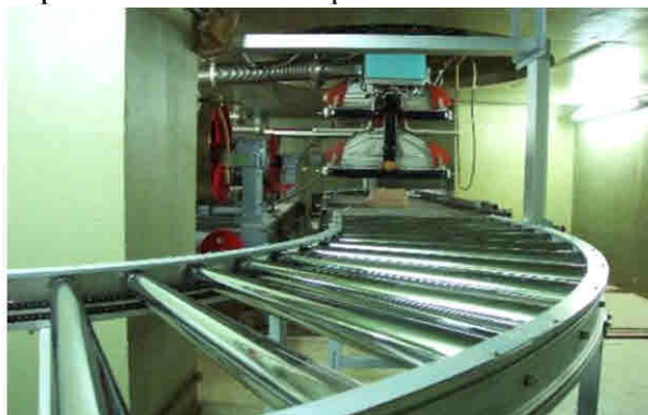
Fig. 1. Electron Beam Processing Section of IRAD, BARC
