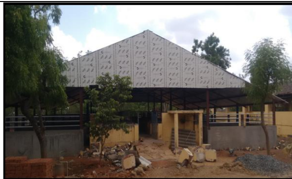
Damage by cyclone
