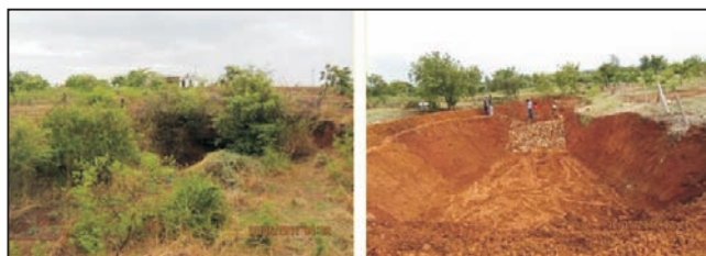
Mini percolation tank at Mirzapur village before (left) and after (right) renovation
