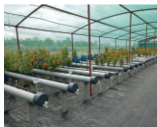
Horizontal sub-surface flow based constructed wetland systems (HSSF-CWs)
