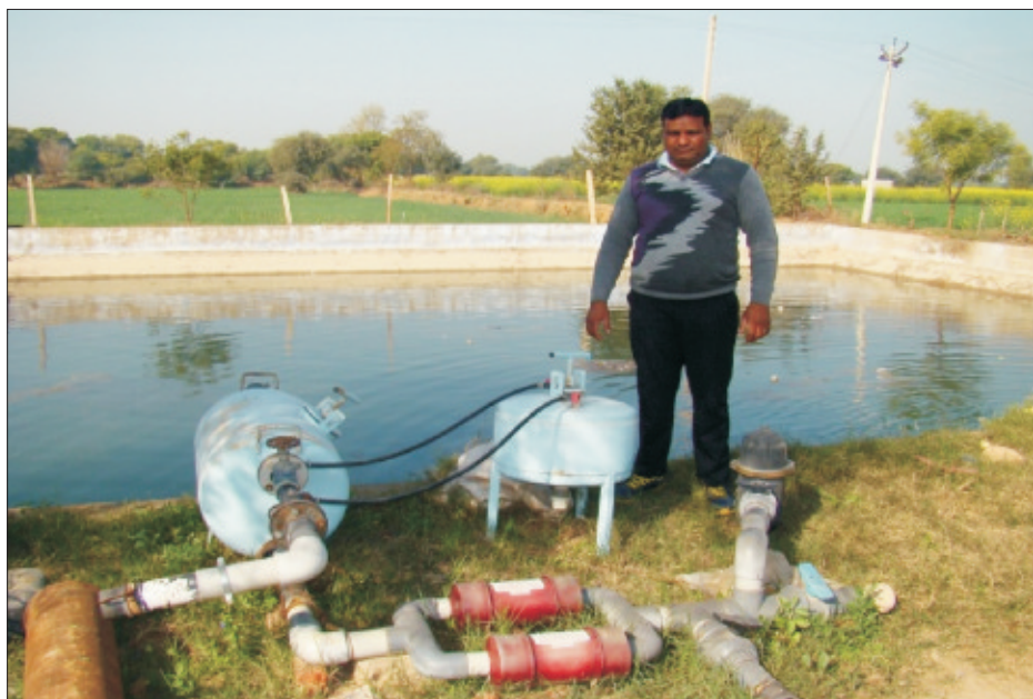
Irrigation pond fitted with drip irrigation system
