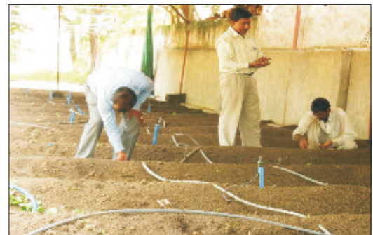
Sprinkler system in vermi compost unit
