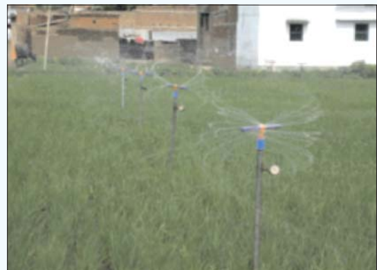
LEWA installed on underground PVC pipe to irrigate rice
