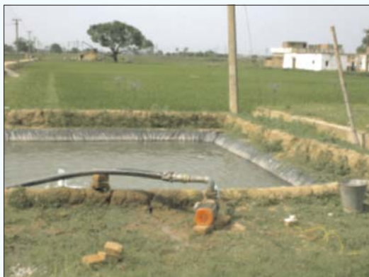
A 1.5-hp prime mover pump (Electric) in operation
