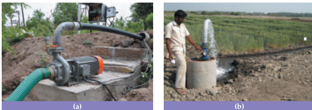
Fig. 2.7. Remotely controlled irrigation pump located 2 km away from NIASM (a), monitoring irrigation with water meter (b)
