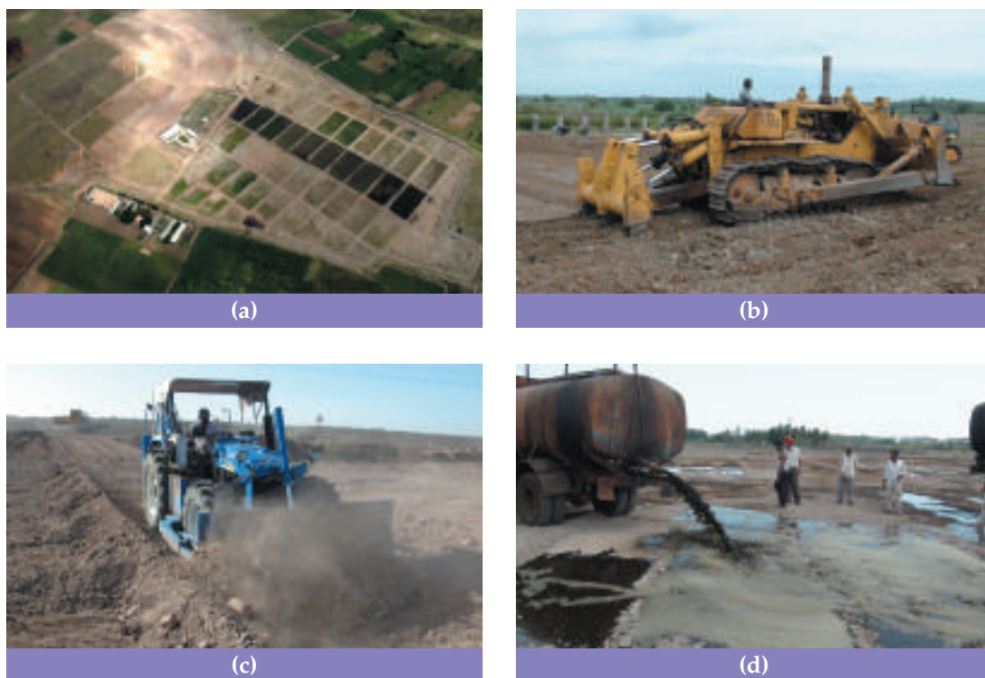
Fig. 2.5. Aerial view of the Research Farm (a), A 350 hp dozer-ripper preparing terraces by ripping and levelling (b), Preparation of farm paths using 75 hp tractor mounted dozer attachment (c), Spent wash being applied for developing research plots (d)
