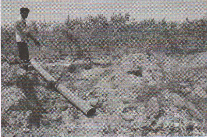
Fig. 5.2. Heavy soil erosion due to breach of earthen field bund
