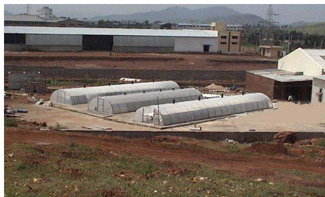
Walk in type solar tunnel dryers installed in M/s Raj Surgical, Village Lakkadvas, Udaipur
