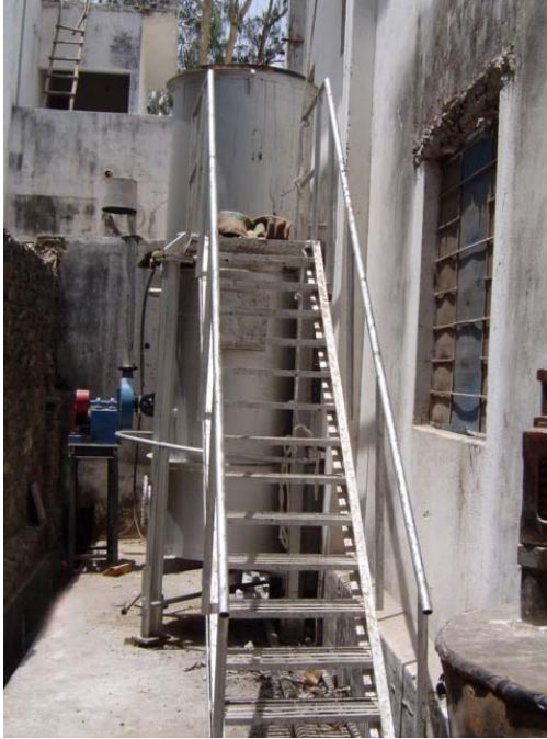
Gasifier system installed at M/s Suman Food Products, Udaipur
