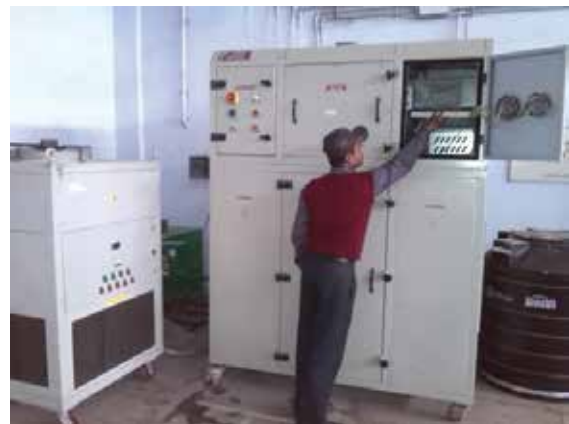
Fig. 31a. Combined drying system
