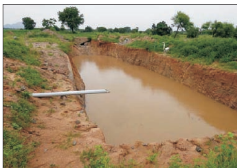
Rainwater harvesting by diverting run-off
