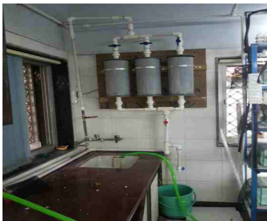
Wall mounted vertical column unit installed in Zebra fish rearing unit
