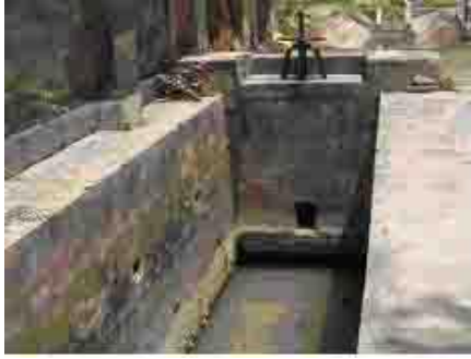
Main sluice gate
