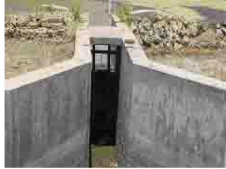
Secondary sluice gates
