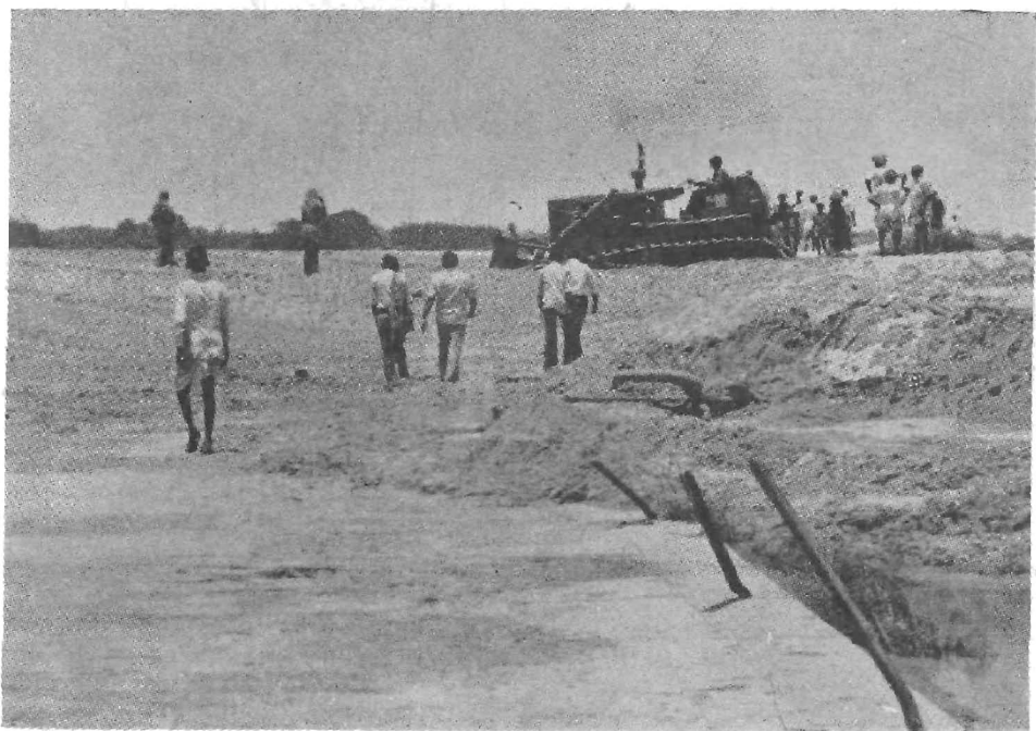
Scene at the Luni causeway on the Jodhpur-Pali highway. The sand and gravel had piled up as high as 3 metres.
