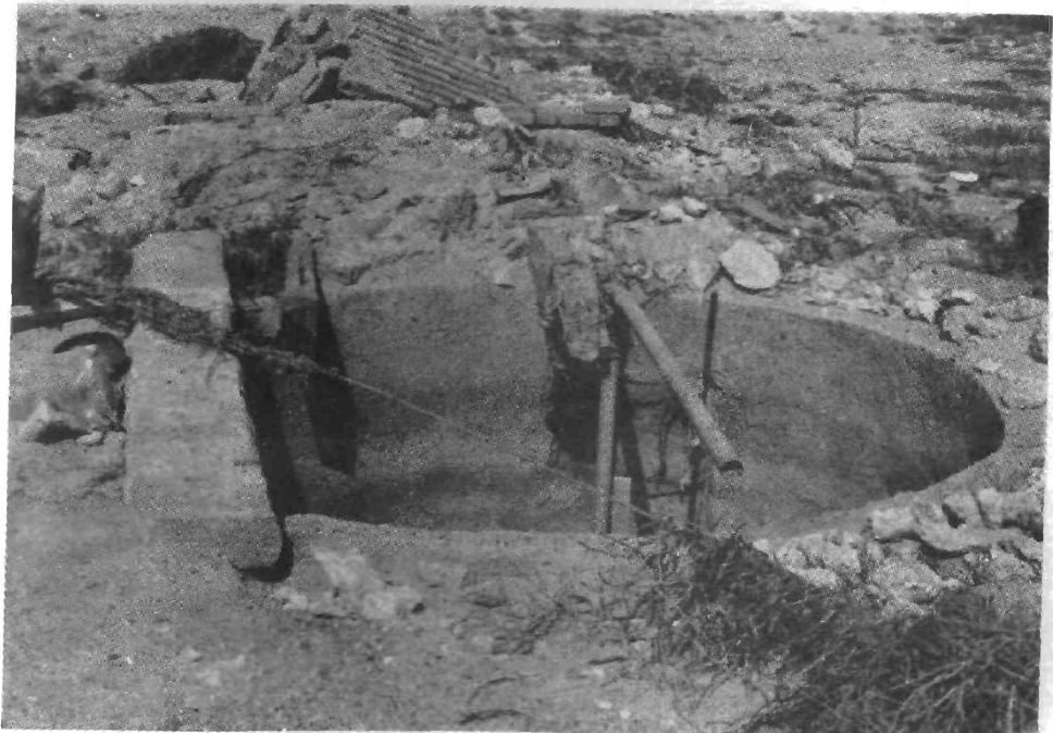
Collapsed structure of an irrigation well. Nearly two thousand five hundred wells together with the irrigation infrastructure are reported to have been seriously damaged.
