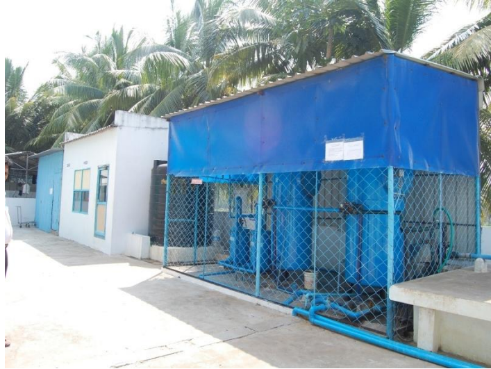
Fig: 05-Water treatment area
