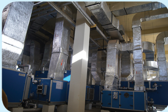
Air Handling Unit of HVAC system
