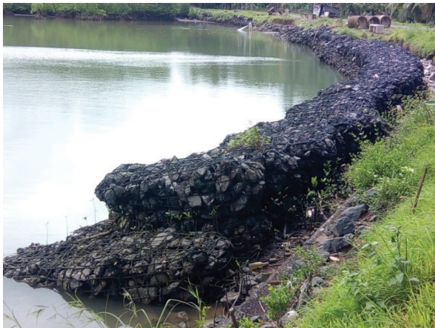
Fig. 3 Gabion structure erected along the coast after tsunami for protection at Chouldari, ANI (Source: B. Gangaiah)
