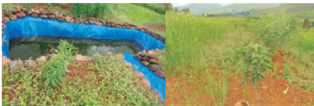
Photo 5.5: Silpauline lined pond for rainwater harvesting to provide protective irrigation to mango plantation
