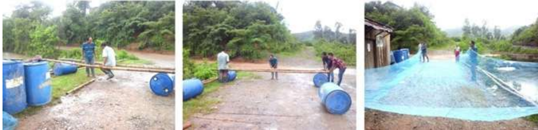
Fig Fabrication of cage for cage culture demonstration at Nungbrung Village, Imphal East District
