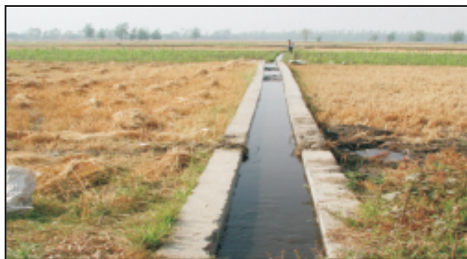
Irrigation channel carrying paper mill effluent for irrigation
