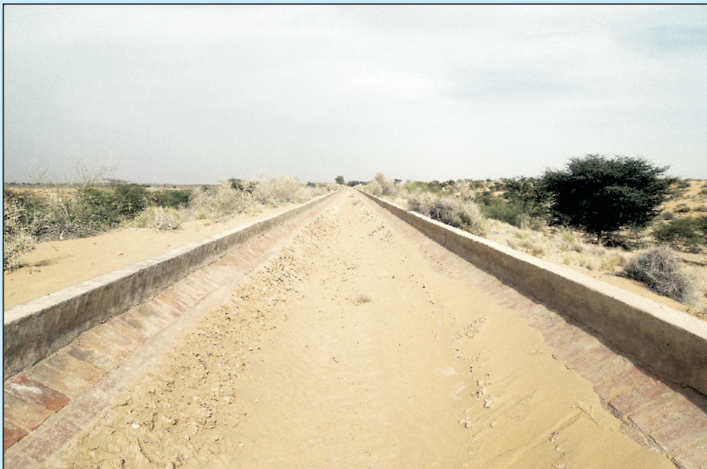
Wind deposited sand in a branch of IGNP: Pre-project severity was more
