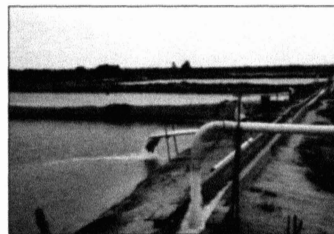
Water intake system
