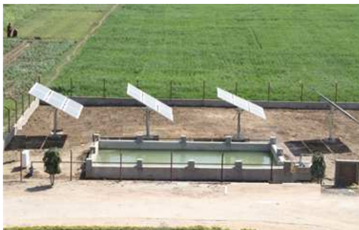
Fig 1. Solar Pumping unit at ICAR Research Complex for Eastern Region, Patna, Bihar
