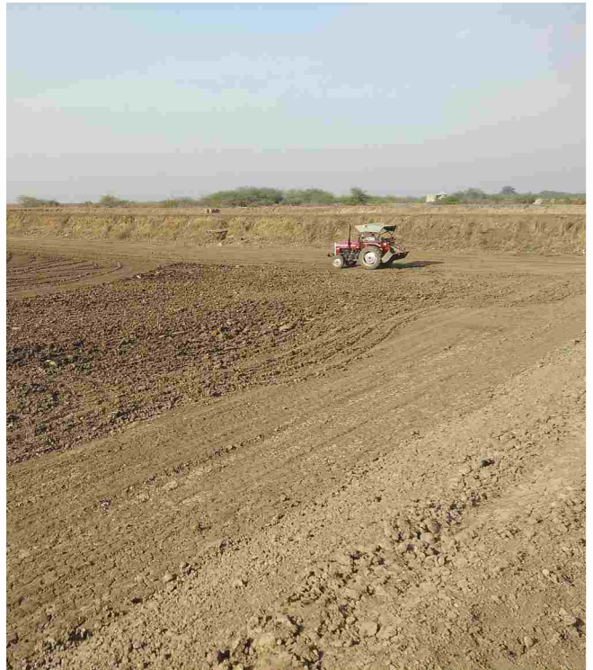
Rectangular earthen pond
