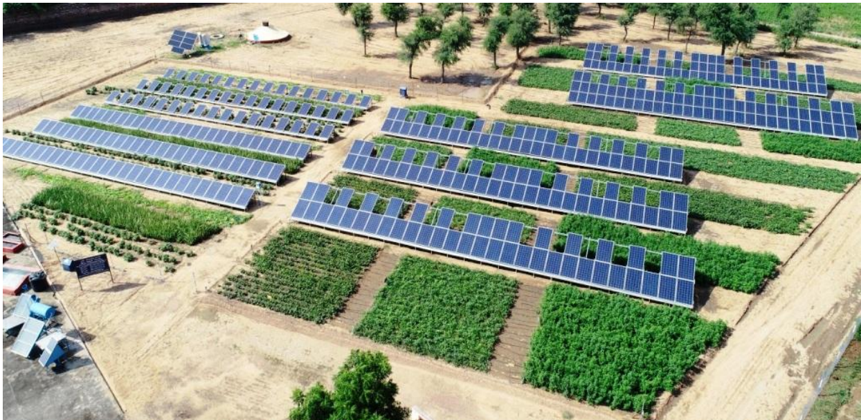
Fig. 2. Installed agri-voltaic system at ICAR-CAZRI, Jodhpur, India
