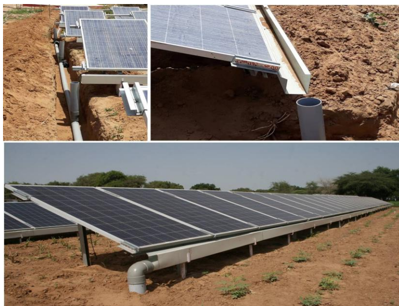
Fig. 7. Rain water harvesting system from top surface of PV module
