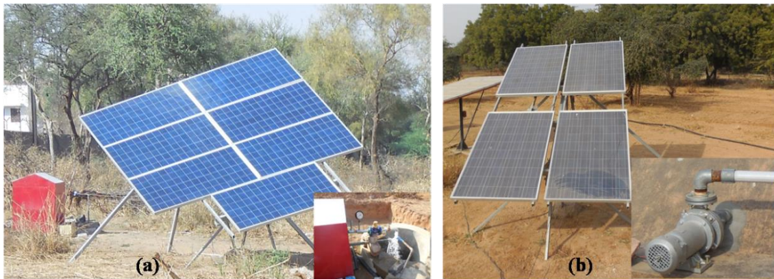
Fig. 1: solar photovoltaic pumps at experimental fields of Central Arid Zone Research Institute, Jodhpur, (a) solar pump with 1 hp AC motor and 7 \times 200 W_p PV array, (b) solar pump with 1 hp DC motor and 4 \times 230 W_p PV array.
