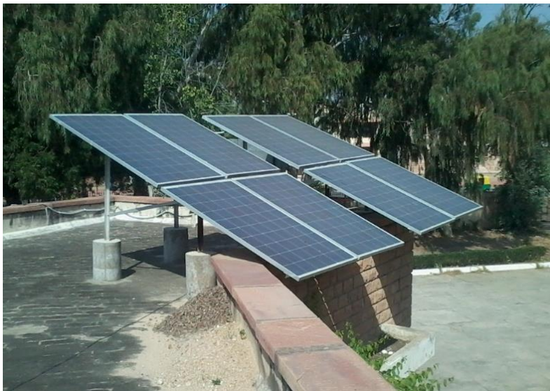
Fig. 1: Roof top solar PV system installed at ATIC building, ICAR-CAZRI Jodhpur (Capacity: 2 kW)
