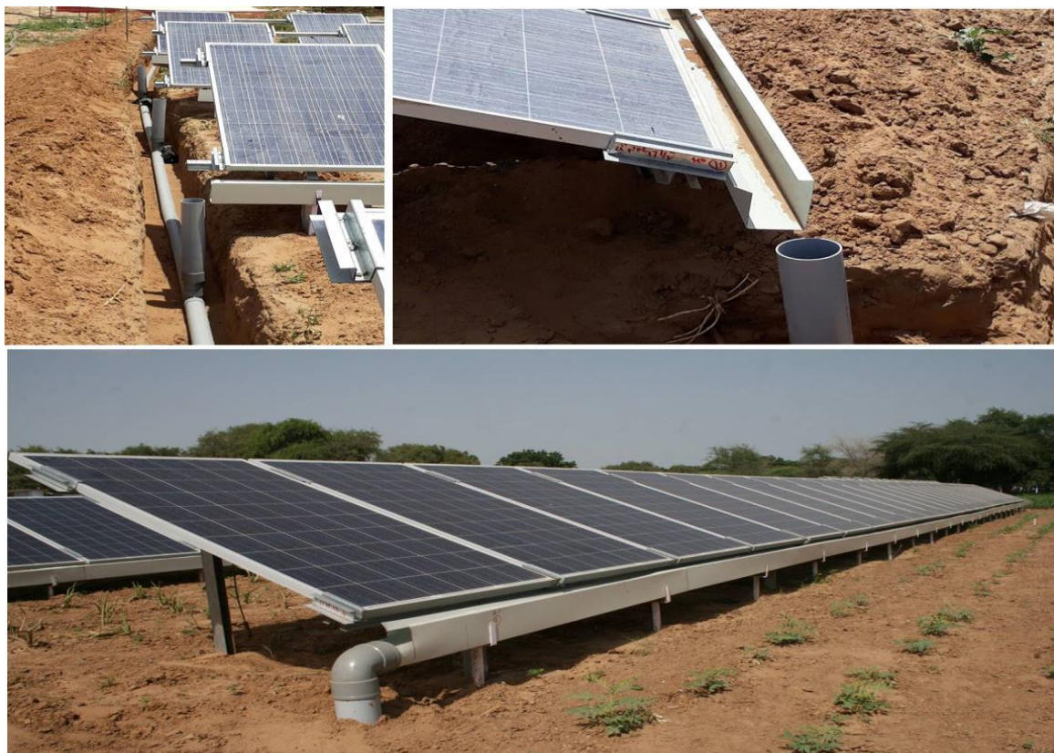
Figure 7: Rain water harvesting system from top surface of PV module
