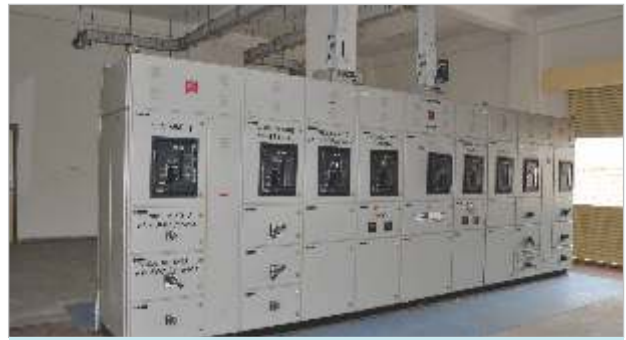
Electrical Substation equipment
