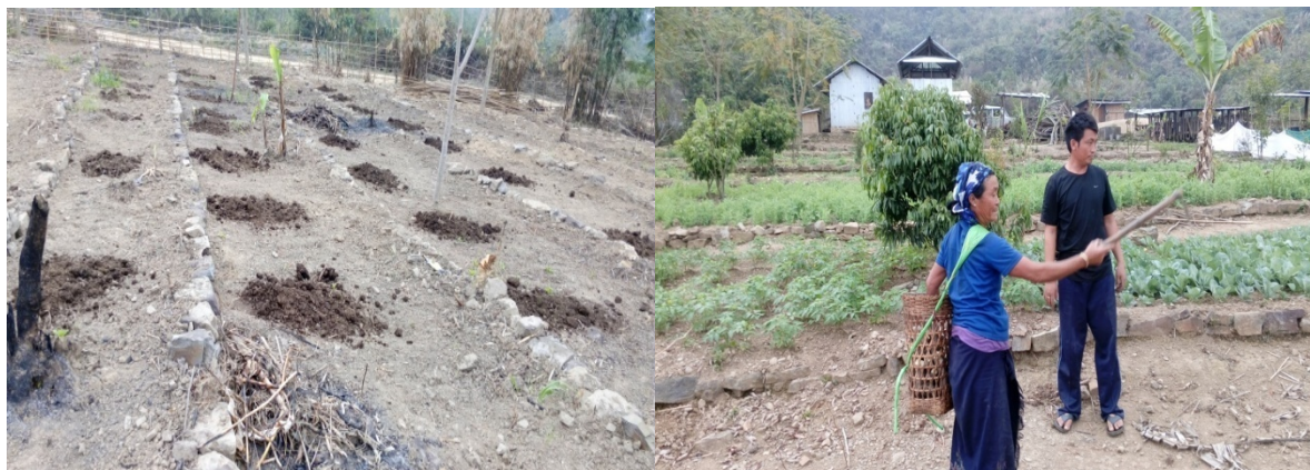
Fig.1 Construction of terraces for SWC. Fig.2 Cultivation of winter vegetable as 2 nd crop in terraces
