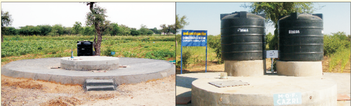
Fig. 15. Rainwater harvesting tank with passive drip system.
