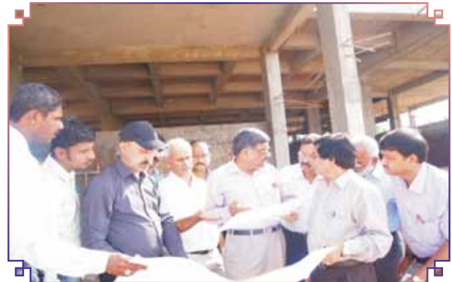
Dr. K. M. L. Pathak, DDG (AS), ICAR, New Delhi interacting with Director and Scientists of NIVEDI and Officials of NDDDB to review the progress of Lab and Administrative building at Yelahanka, Bengaluru on 24 th October, 2013.
