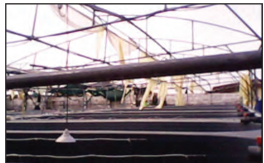
Damage to shrimp hatchery due to Cyclone Phailin
