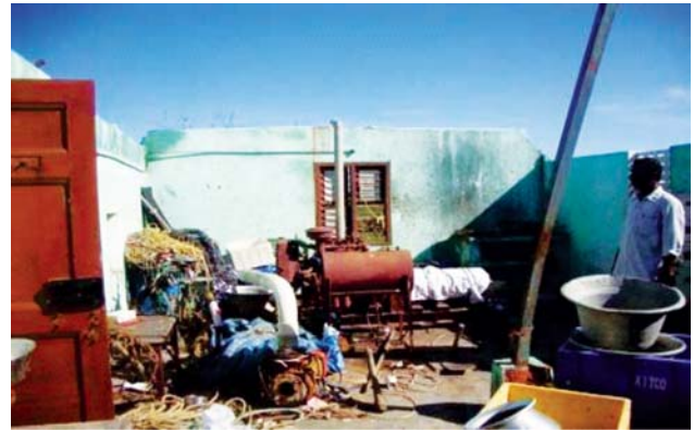
Infrastructure damage to shrimp farms - Nanamedu
