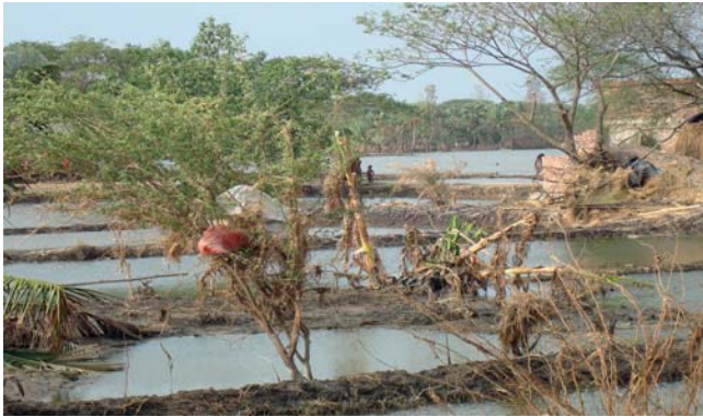
Damaged pond dykes due to Aila Cyclone at Chunakhali, Basanti
