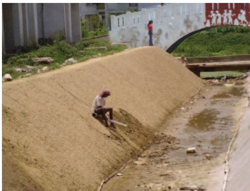
Fig 2 : Placing of jute-PP union fabric and covering by a layer of top soil
