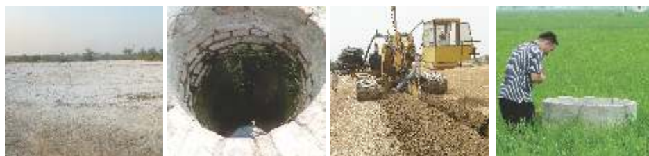
Fig 2.1. Waterlogged saline soil (left), installation of SSD system (third), post-project bumper wheat crop (right)
