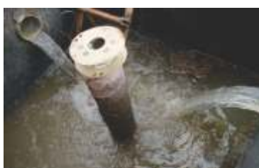
Fig 6.2. Working of renovated groundwater drainage cum recharge structure
