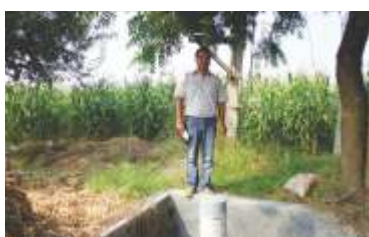
Fig 6.1. A renovated groundwater drainage cum recharge structure
