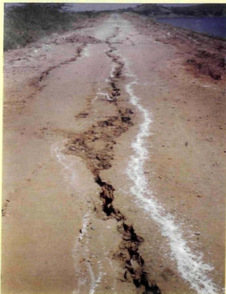
Plate 10. Large cracks developed on the Kesawati river dam
