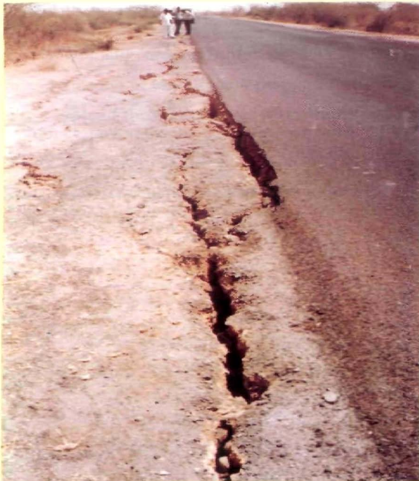
Plate 4. Long cracks developed along Bhuj - Bhachau road near Sikra village
