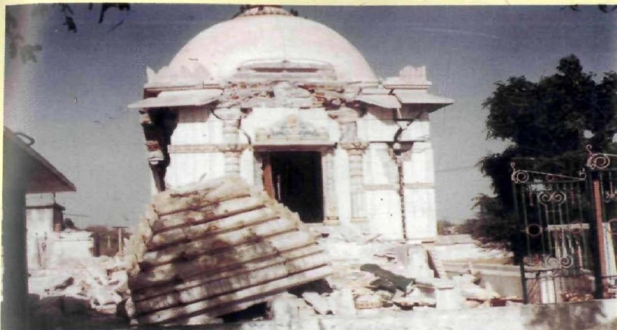
Plate 9. A severely damaged temple near Gundala village (Mandvi taluk)
