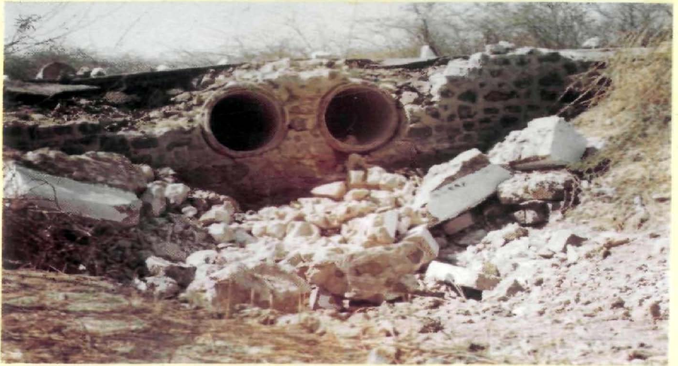
Plate 11. A badly damaged culvert near Sikra village
