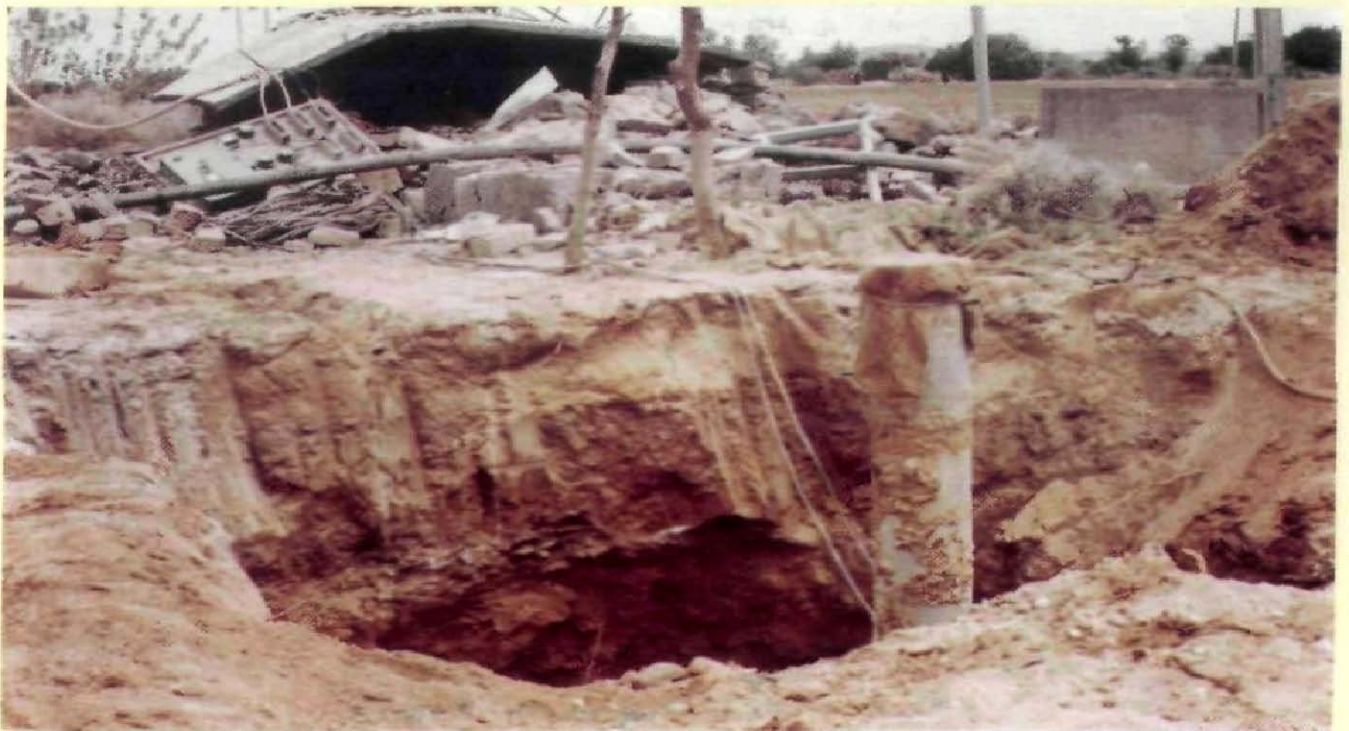
Plate 12. Damaged irrigation well near Manfara village
