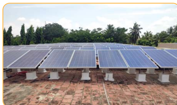
Fig. 84: Roof top solar system
