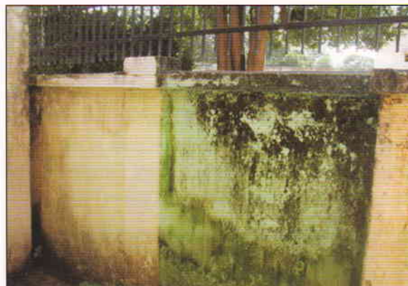
Fig. 47. Fungal effect on shellac emulsion coated wall and commercial paint coated wall
