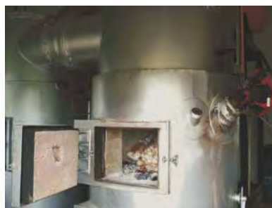
Incinerator for burning the infected lab waste with environmental protection
