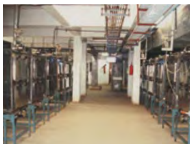
Air-handling unit is equipped with HEPA filtration of the outgoing air.
