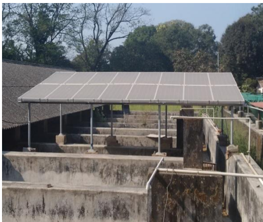
Solar power plant
