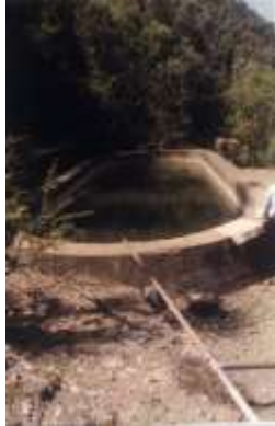
Spring water harvesting through concrete lined tanks in Moolbury Watershed of Himachal Pradesh
