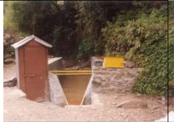
The HI Flume, Stilling Well and Housing for Stage Level Recorder
