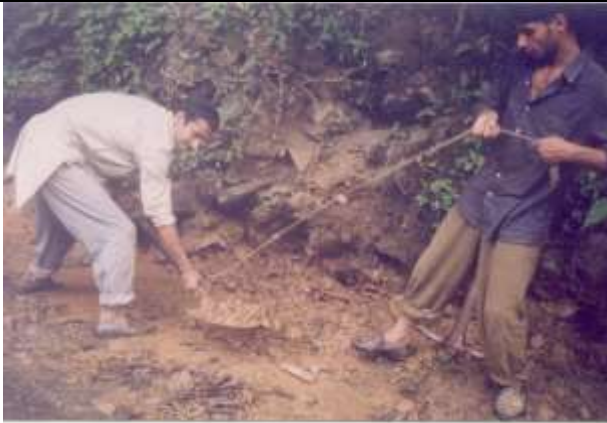
Work in progress for construction of the channel for installation of HL Flume
