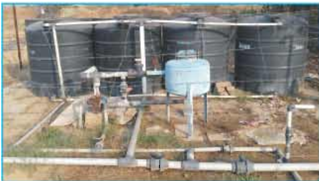
Desalination system for water
