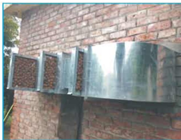
Guar straw ball based dehumidification system for evaporative cooled room
